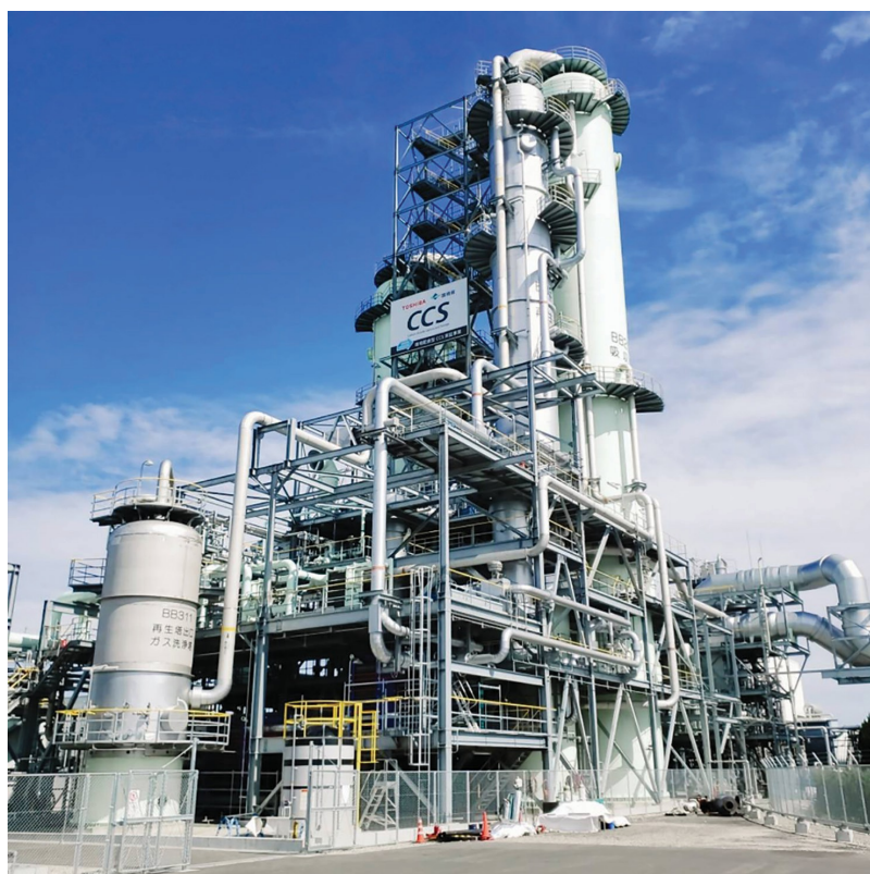
This large-scale pilot plant for carbon capture went into operation in 2020 in the Japanese city of Mikawa at the local biomass power plant. The power plant is fired with palm kernel shells as its primary fuel and has a capacity of 50 MW (photo: Toshiba ESS).
